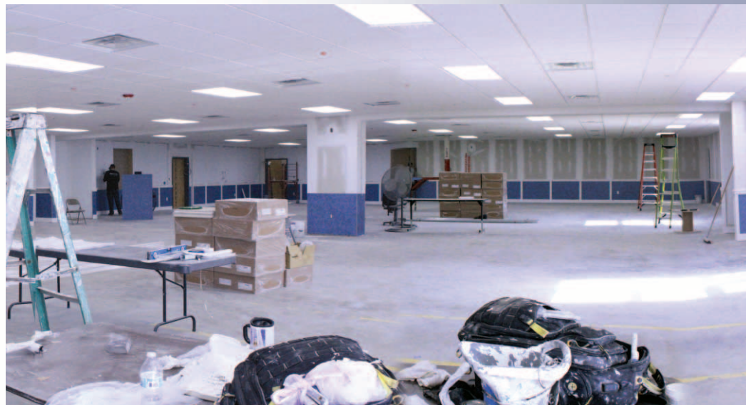
Phase one of KSI's Skill Development Center renovation began in summer of 2023.
