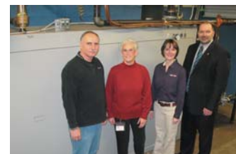
Pictured with the new boiler are (left to right) KSI's Shawn Bowman, Discover Bank's Sherry Berman and Amy Walls, and KSI CEO, B. Craig Crouch.
